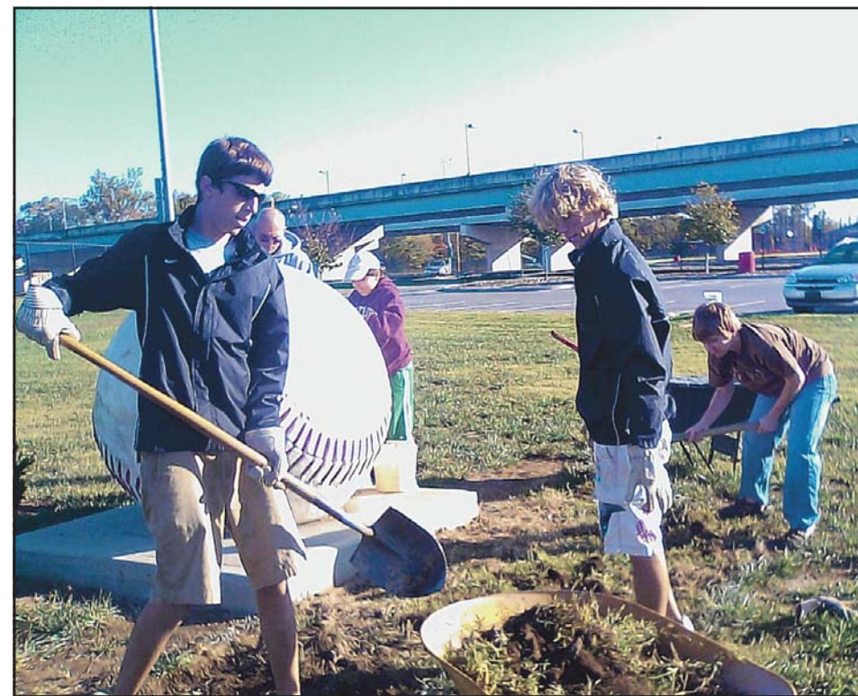
Chris Jack (standing, right) refurbished the concrete baseball at Domtar Park for his Eagle Scout project.
